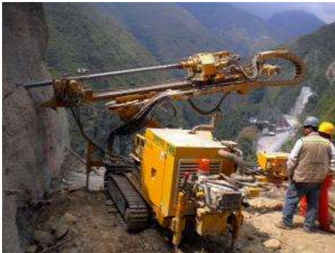
Example of a poor working platform
