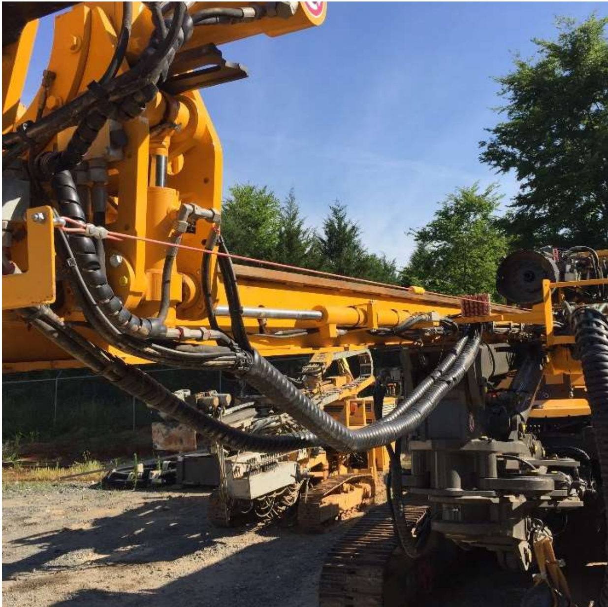
Trip Device parallel to mast
