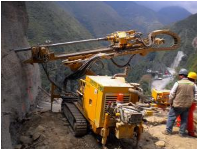
Example of a poor working platform
